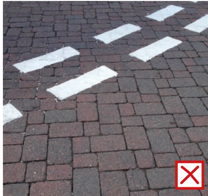
No white lining to block paving.
