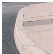
Pre-cast concrete kerb
