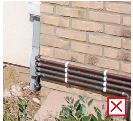
Pipework clearly visible from the street scene is not acceptable
