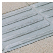
Tactile corduroy paving
