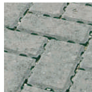
Permeable keyblock paving
